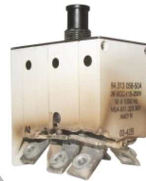
Overheated 50Amp CB
