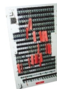
CB panel used in emergency electrical power distribution system
